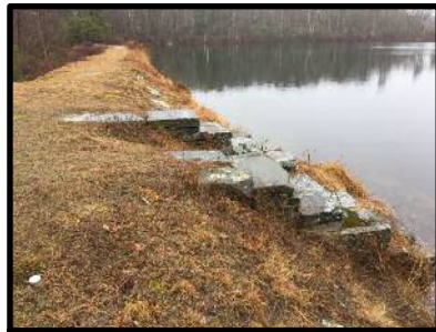
Southeast Dam and Relict Spillway of Wolf Lake. All Lake Outflow is now West to the Neversink River.
