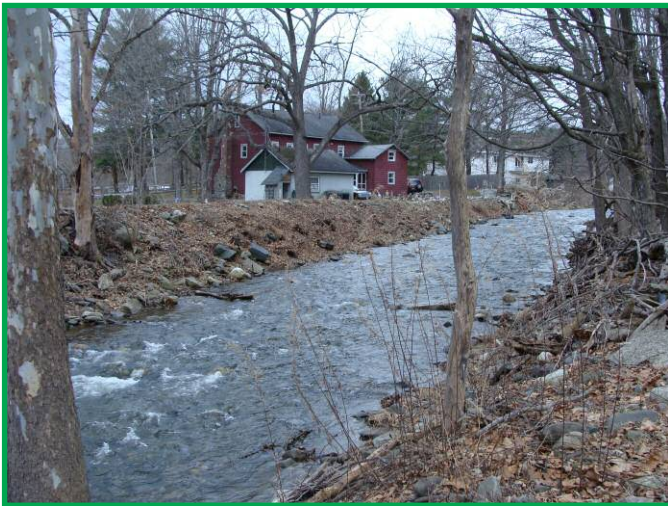
Location A. Channel fill material bermed up against backyard on stream right. Looking upstream.
